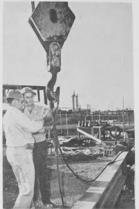
A CRANE is hooked to one end of the bridge's truss section under the supervision of T. O. Lucas, transportation zone foreman. Two cranes lifted the fourteen-ton bridge.
